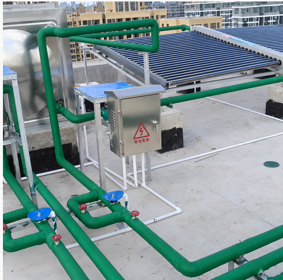
Rooftop hot-water equipment and pipework
