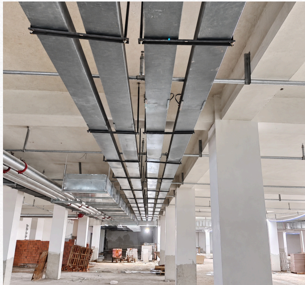
Basement cable trays and service installation
