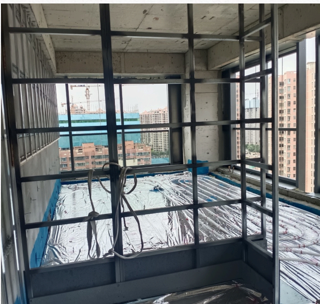
Light-gauge steel partitions
